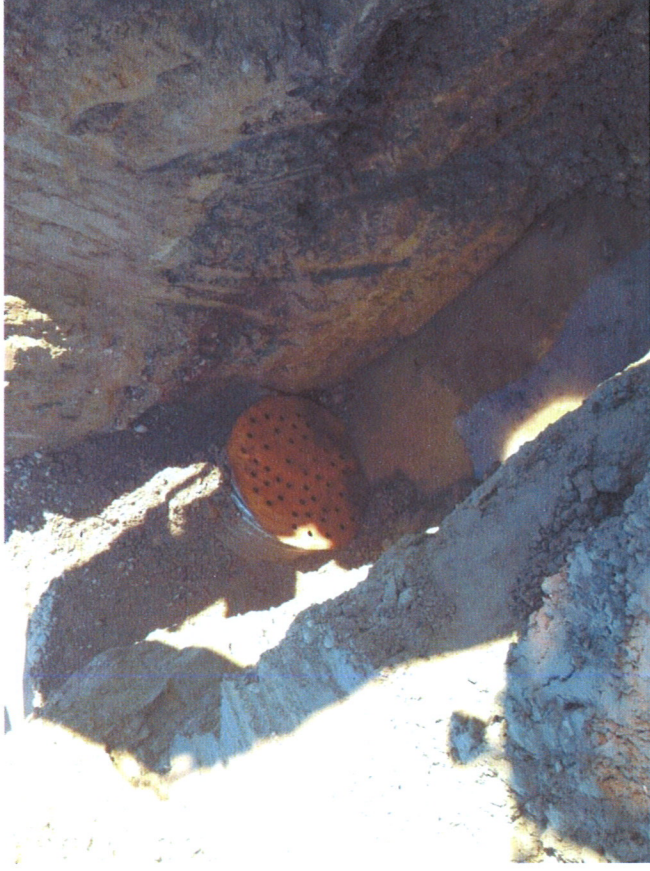
Looking down on the end of the newly installed 40 foot section of pipe, The next 20 foot section of pipe would be installed the following day.
