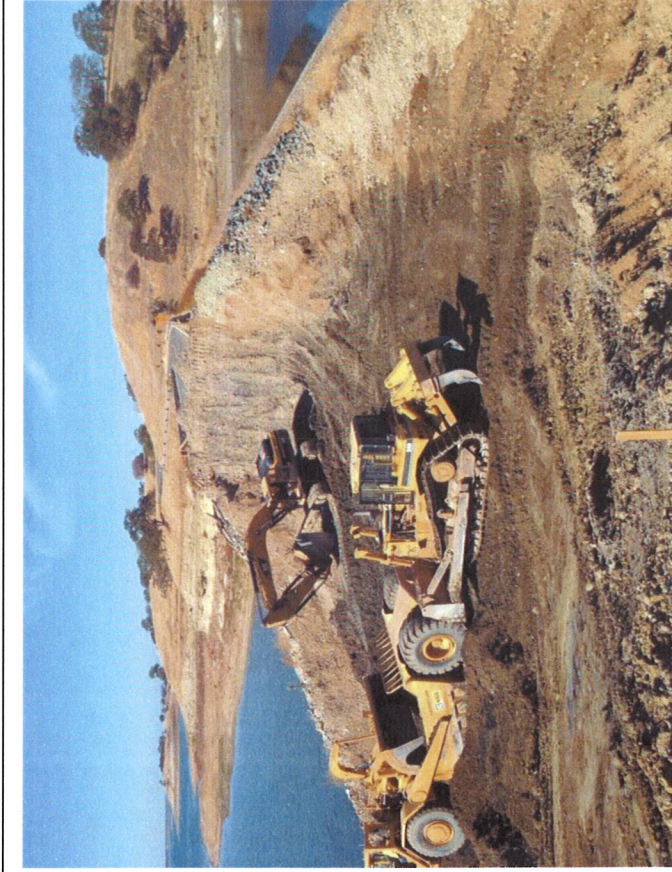
Looking west on the Causeway - Contractor excavating Causeway. The dark material is random material (dirt), which comprises the core of the Causeway. The light material on the right of the photograph is drain zone material (river rock and cobble), which comprises the outerlayer of the Causeway.
