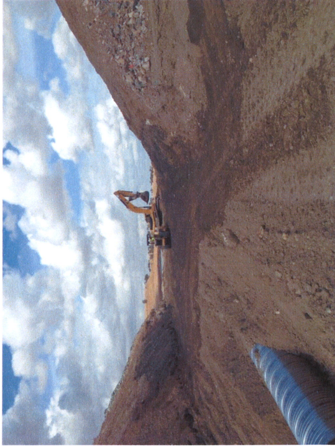
Looking north towards Rabbit Creek. Pipe is installed and backfilled. Preparations for reconstruction of the Causeway are underway.
