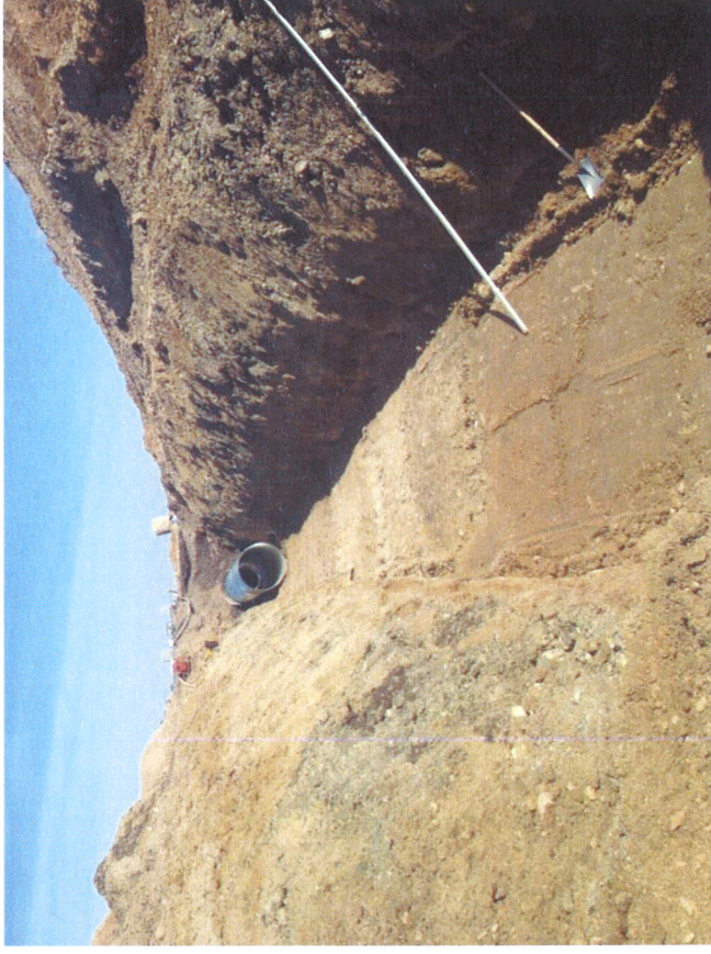
Looking north down the dry trench. The remaining pipe section were installed that day.
