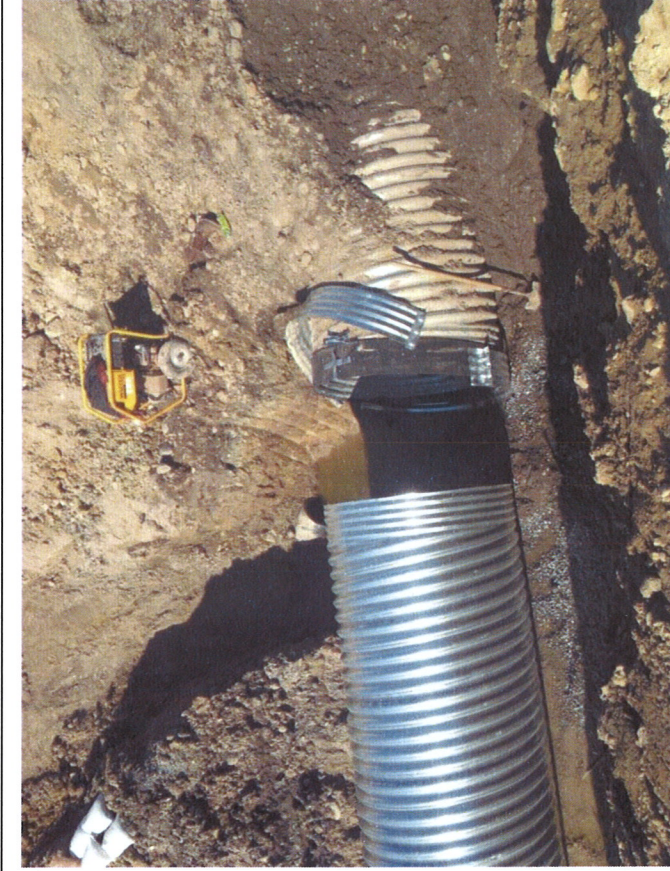
Looking down on the pipe end at the bypass drain. The drain remains effective and next pipe section is placed for installation.
