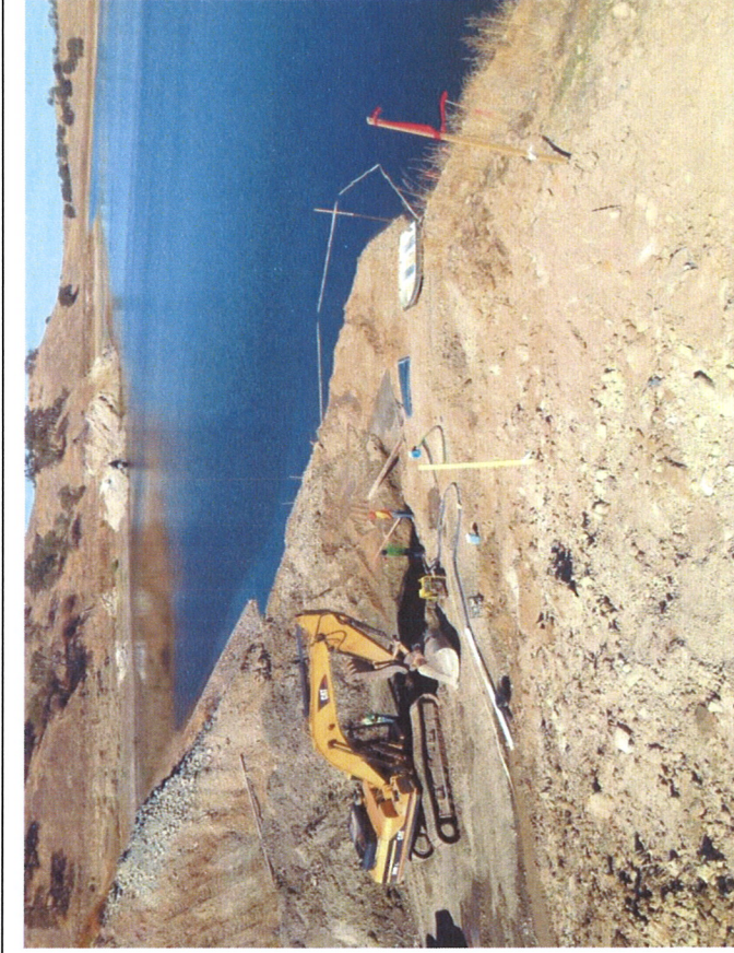
Looking northwest from Causeway towards Rabbit Creek - First 40 foot section of pipe installed with concrete backfill to seal seepage from Rabbit Creek
