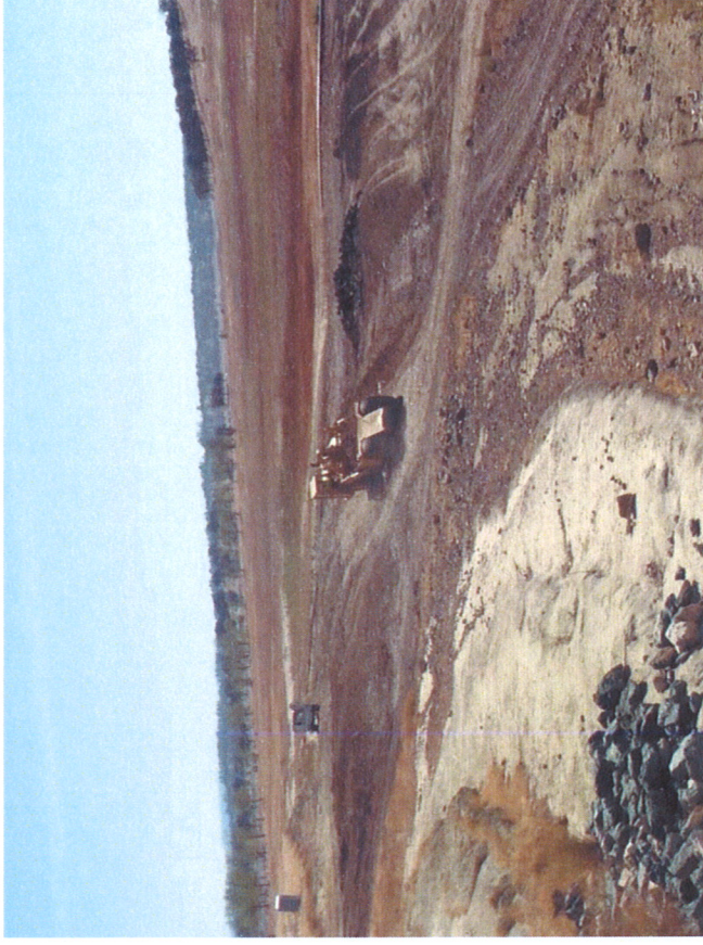
Looking south from Causeway - Scraper hauling and sorting engineered fill material excavated from Causeway to stockpiles. On the left, drain zone material (river rock and cobble). On the right, random material (dirt).
