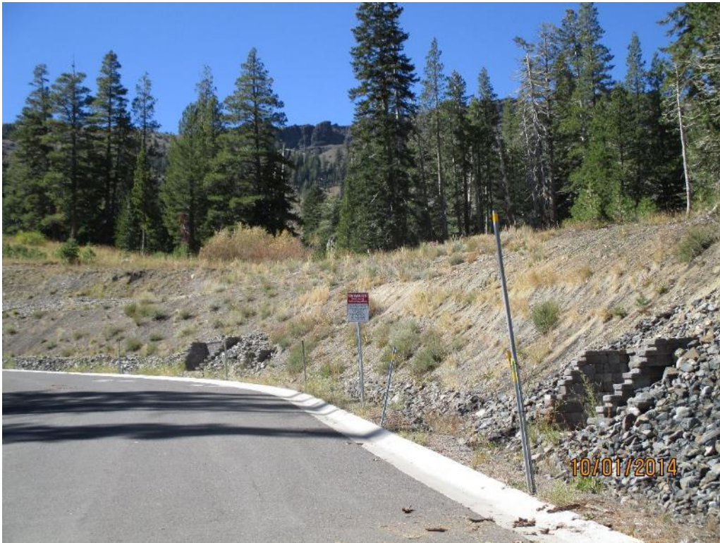
Photo 9. Temporary slope stabilization within Palisades 5. Success of temporary revegetation is variable, but over slope stability maintained by erosion control fabrics and rock as evidenced by lack of dirt and debris on road.
