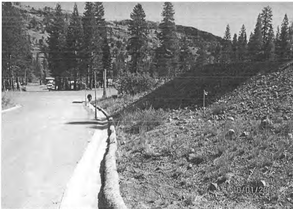
Photo 1. Examples of erosion control material in place during construction of Timber Creek Phase 1.
