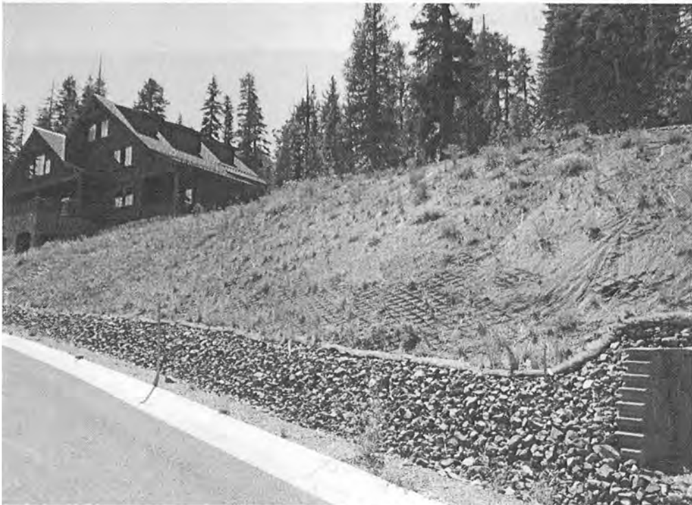
Photo 8. Temporary slope stabilization within Palisades 5. Success of temporary revegetation is variable, but over slope stability maintained by erosion control fabrics and rock as evidenced by lack of dirt and debris on road.
