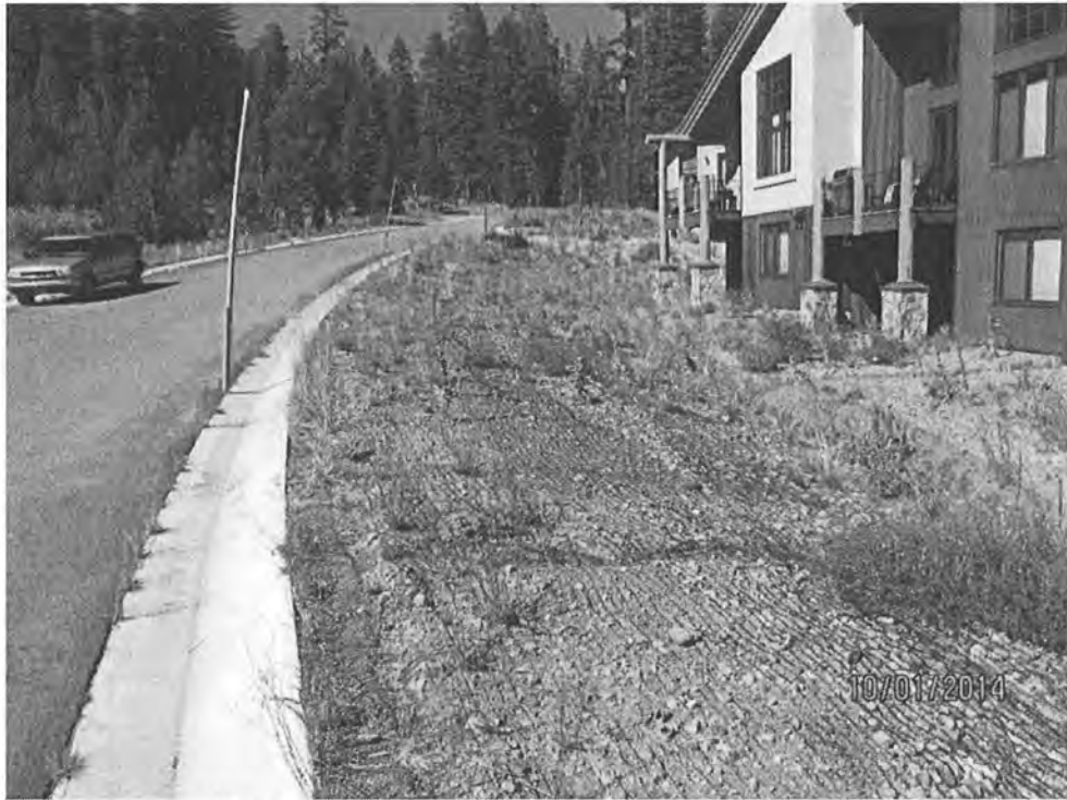
Photo 11. View of failed revegetation along Sentinels Way.
