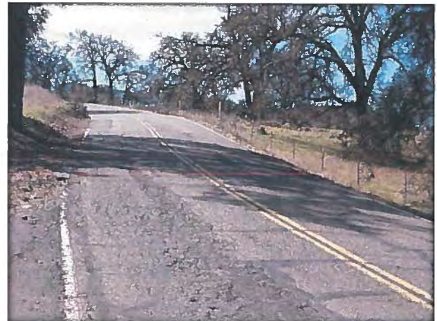
Figure 6- Stony Creek Curve with No Signage and Worn Pavement
