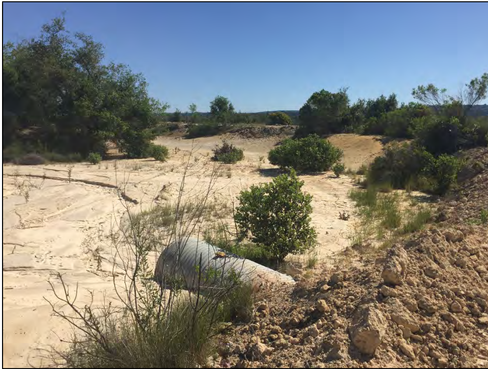
Photo 3: Looking northeast at culvert under road. Signs of sediment deposition from upslope mine spoils. Dominant vegetation: sandbar willow ( Salix exigua ), arroyo willow ( Salix lasiolepis ), whiteleaf manzanita ( Arctostaphylos viscida ), yerba santa ( Eriodictyon californicum ), toyon ( Heteromeles arbutifolia ), coyote brush ( Baccharis pilularis ), interior live oak ( Quercus wislizeni var wislizeni ), chamise ( Adenostoma fasciculatum ), Ponderosa pine ( Pinus ponderosa ), Himalayan blackberry ( Rubus discolor ).
