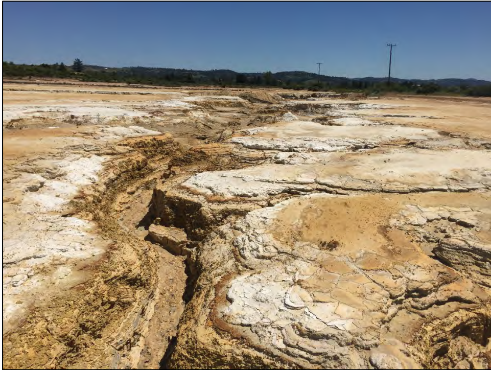
Photo 15: large area of reel and gully formation from channel flow. Highly erodable sediment deposits from mining activity. No vegetation in the area.
