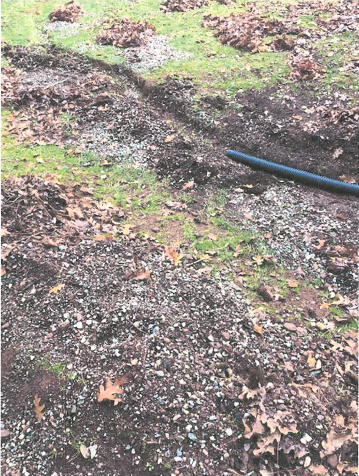
Another photo of debris, sediment and driveway rock/gravel in my backyard resulting from culvert and ditch drainage failures.
