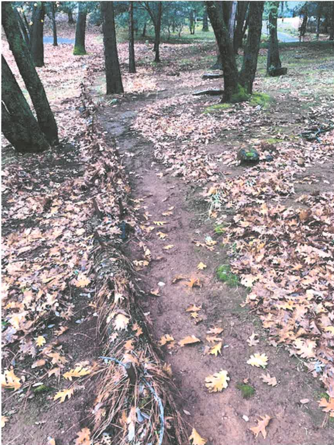
This 75 feet of wattle was installed 5 years ago as a second line of defense against culvert and ditch failures on Robin Lane. Both the ditch and wattle structure are to convey road runoff beyond the foundation of my house.
