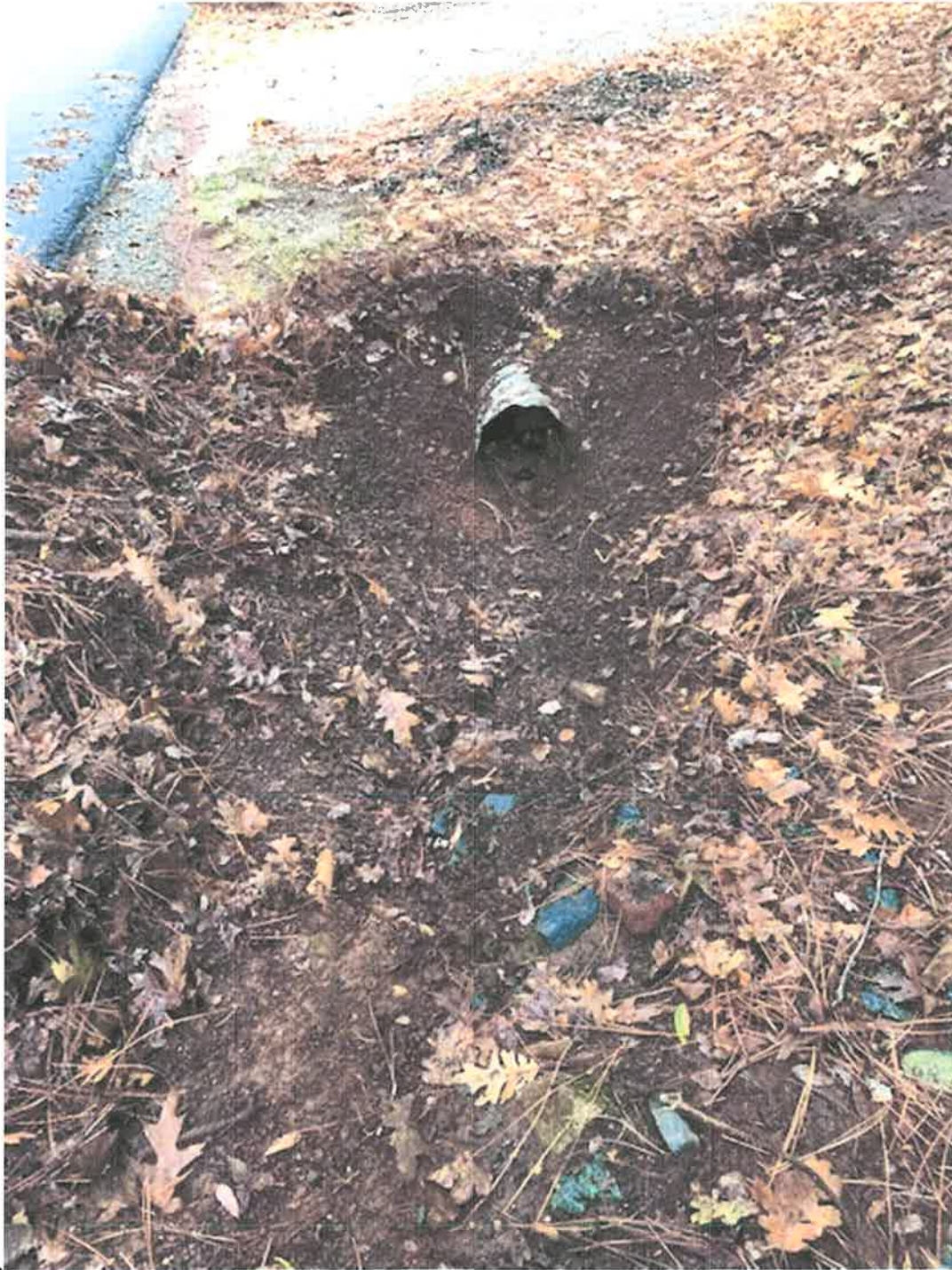
The second culvert I have cleaned out repeatedly for many years to guard against plugging and subsequent ditch failure.
