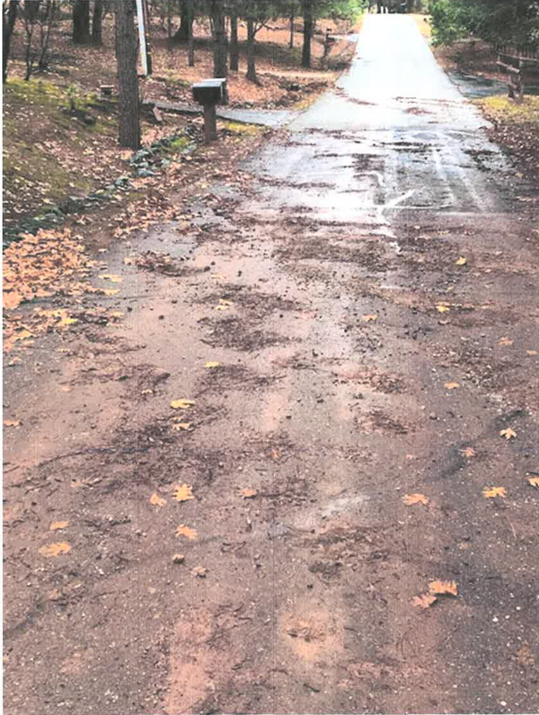
Robin Lane after 12/7/19 rain storm. On the left side of the photo you can see where the ditch system was not able to handle storm runoff (failed). This type of event has reoccurred on Robin Lane for many years. To my knowledge PACSD RZ1 has never cleaned this type of road damage up. This is a safety hazard to both pedestrians and vehicles. You can see further up Robin Lane in the photo where the failed culverts led to large amounts of runoff and debris to cross Robin Lane ultimately impacting my property (follow the brown debris lines).
