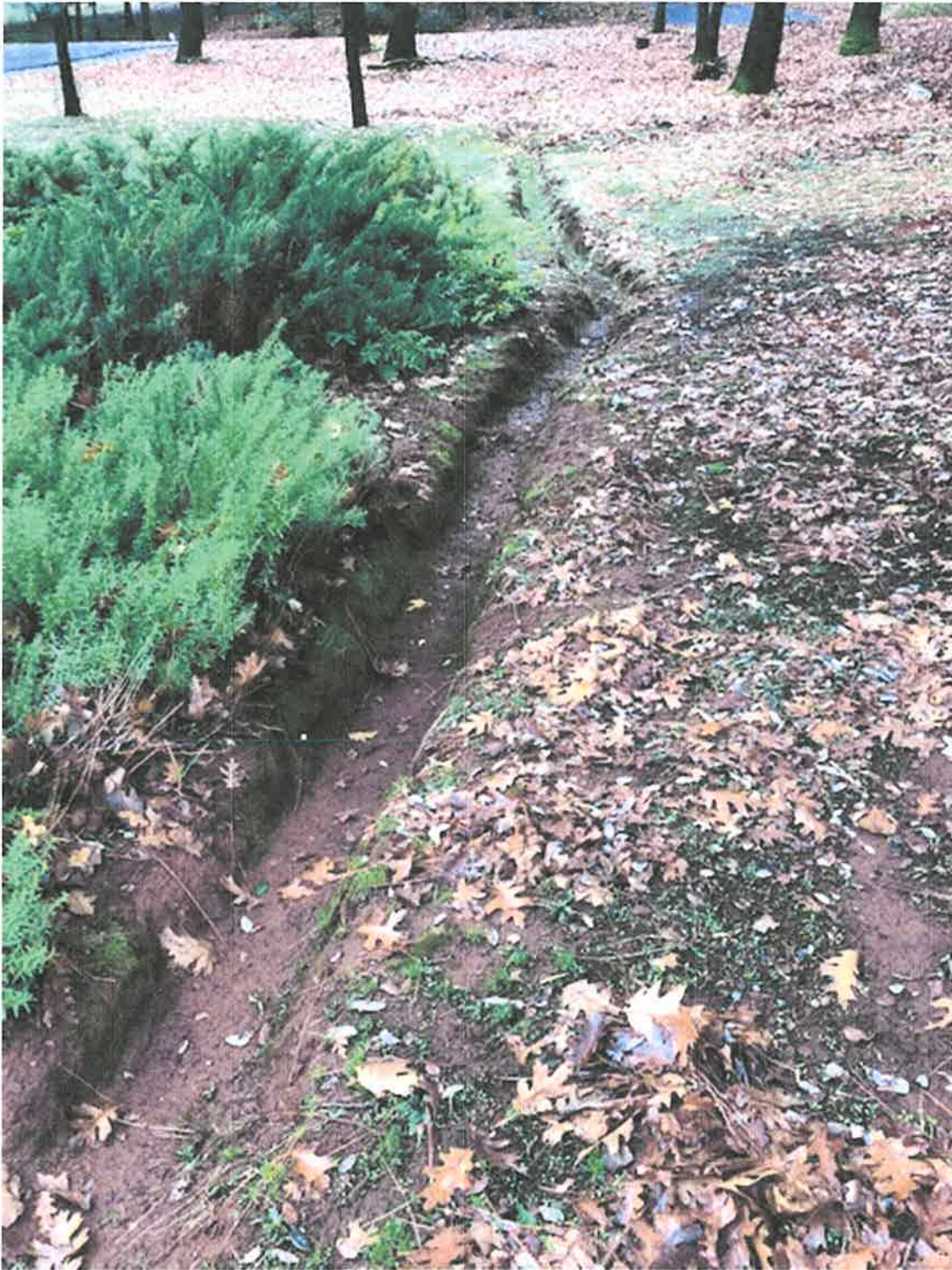
The ditch in my front yard I have maintained for 20 plus years to guard against culvert and ditch failures on Robin Lane.
