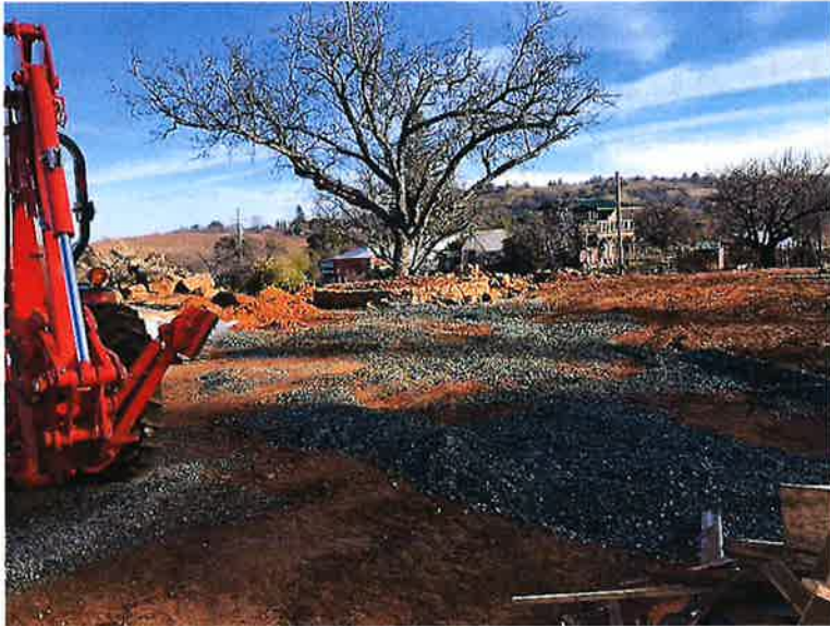
Overview of Project Area showing ongoing construction. Heavy prior disturbance is evident.
