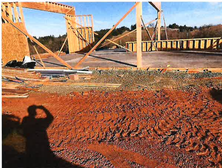
Overview of Project Area showing ongoing construction. Ground disturbance has already occurred and basement is installed. All visible soils are sterile for cultural deposits.
