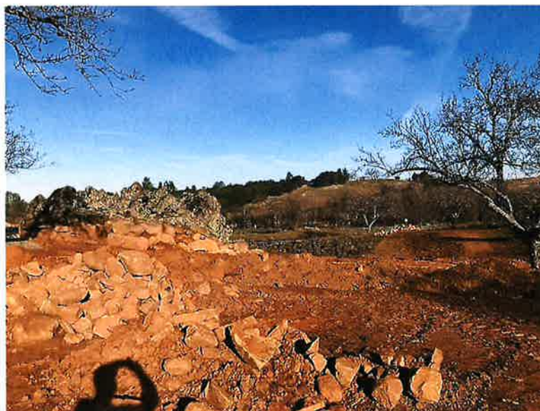
Backdirt from installation of basement. All visible soils are previously disturbed and sterile for cultural deposits.
