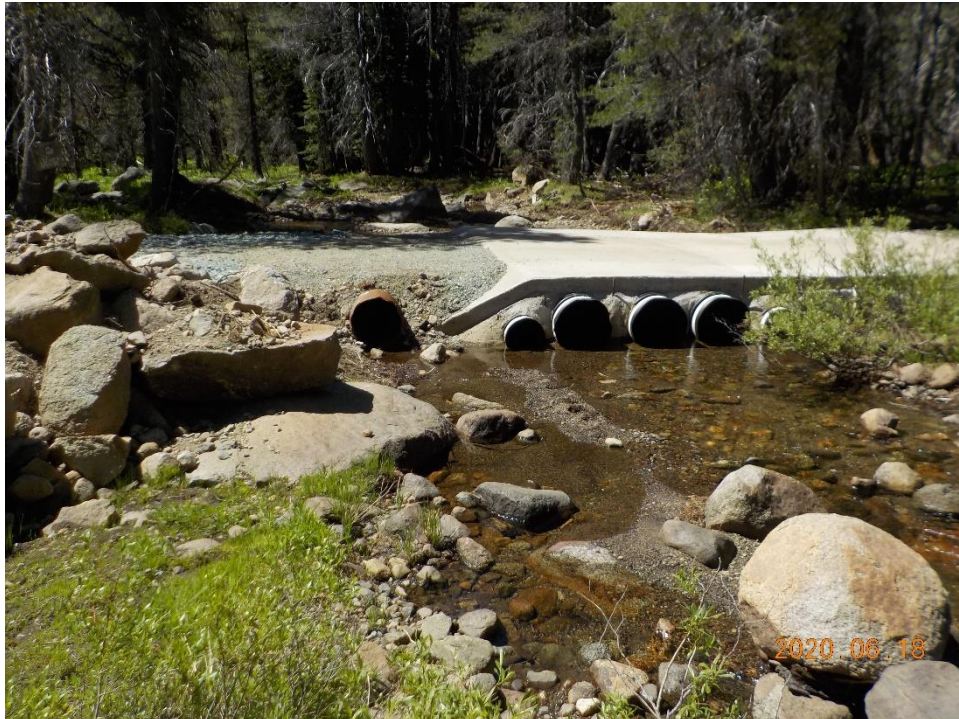
Photo 2. Overview of the constructed crossing with three 18-inch HDPE culverts, two 12-inch HDPE culverts, and one 18-inch CMP culvert; photo direction – south; June 18, 2020.
