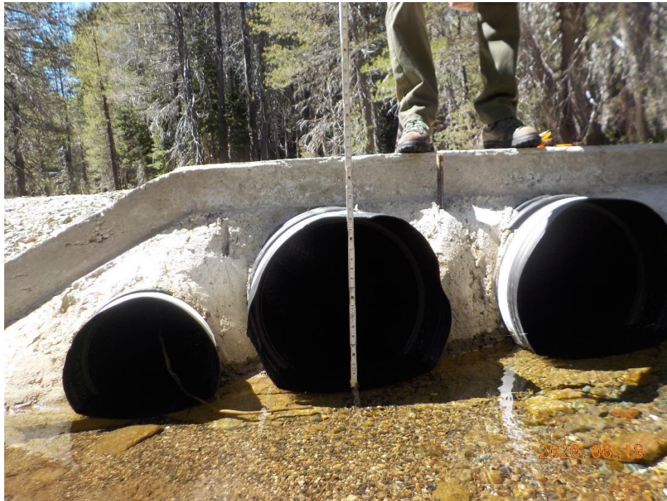
Photo 3. Inlet of 18-inch diameter HDPE culvert incased in concrete and adjacent culverts; photo direction – south; June 18, 2020.
