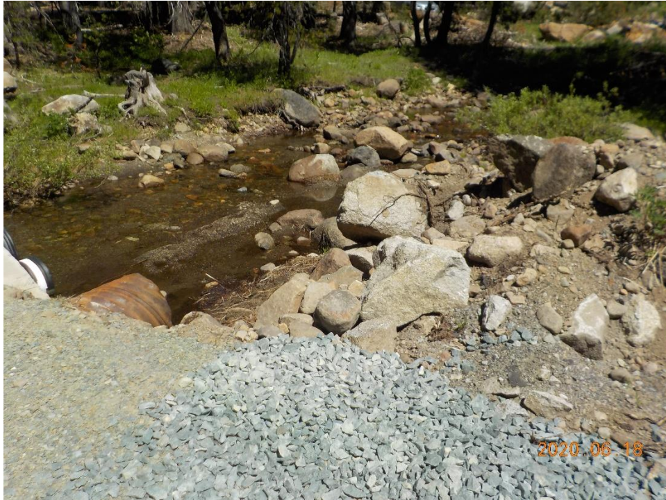
Photo 7. Inlet of 18-inch diameter CMP culvert and loose soils and rocks placed on the left bank of the stream; photo direction – northwest; June 18, 2020.
