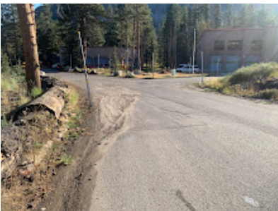
Loop Road Drainage Issue 9.6.22 #3.jpg 1543K
