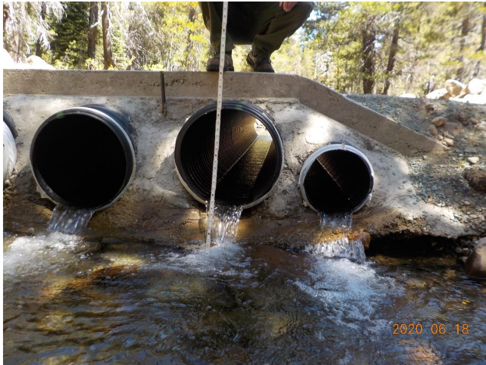
Photo 5. Outlet of 18-inch diameter HDPE culvert incased in concrete and adjacent culverts. Measured culvert is set approximately 13 inches above the streambed; photo direction – north; June 18, 2020.
