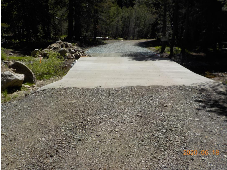
Photo 1. Concrete surface of constructed crossing with estimated 1,350 cubic feet of concrete; photo direction – east; June 18, 2020.
