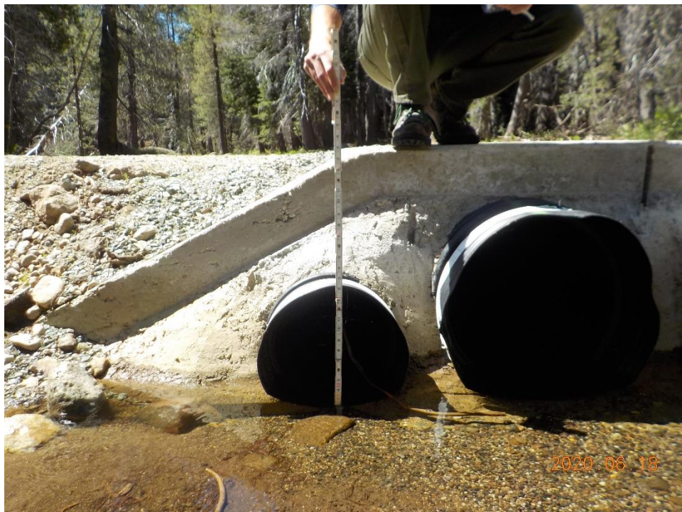
Photo 4. Inlet of 12-inch diameter HDPE culvert incased in concrete and adjacent culverts; photo direction – south; June 18, 2020.
