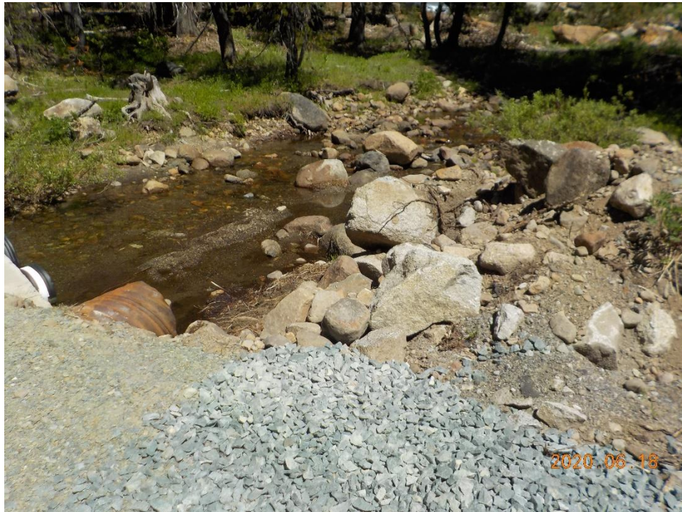
Photo 7. Inlet of 18-inch diameter CMP culvert and loose soils and rocks placed on the left bank of the stream; photo direction – northwest; June 18, 2020.
