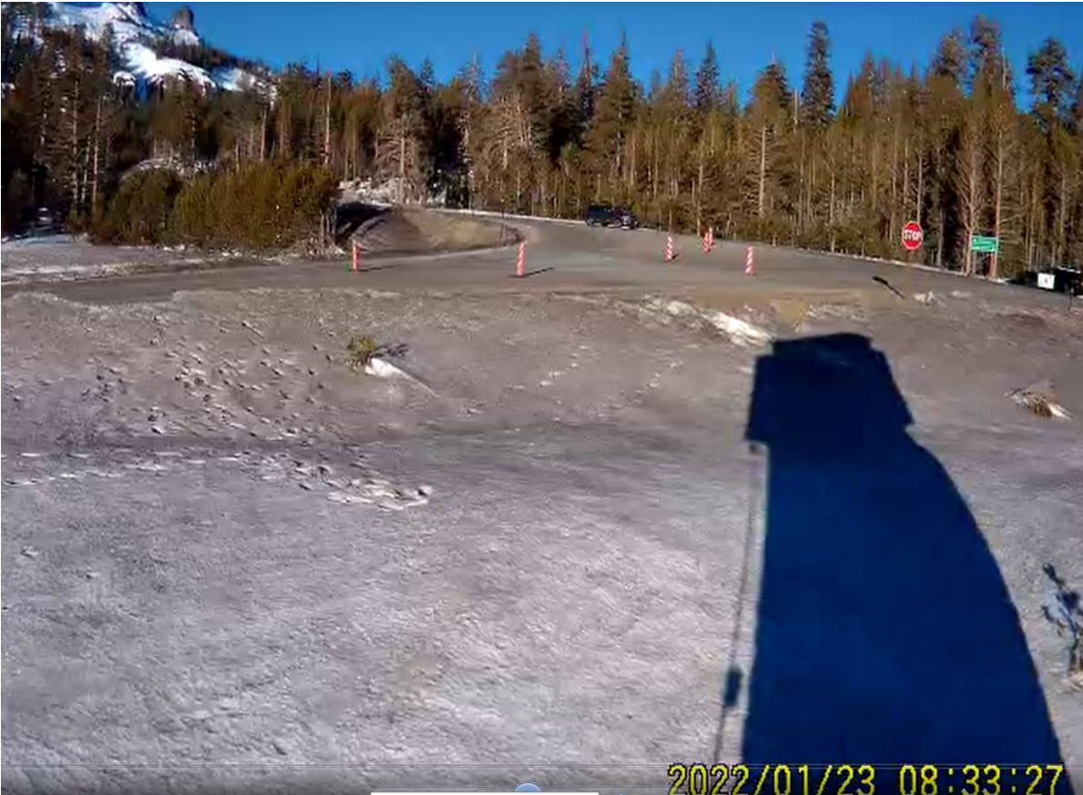
SR 88/KMR still free-flow at 8:33 AM. Coning pattern in place. Officer present, not assigning ROW.
