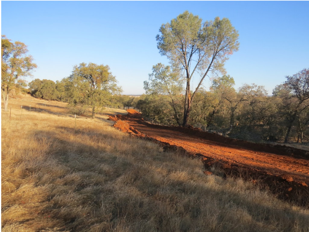
Photograph 11: A recently graded access road in the eastern portion of the project site; adjacent to oak woodland savannah.
