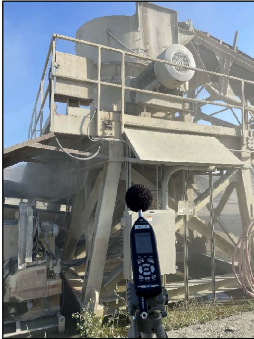
Figure 9 – Crusher GP500 before curtains
