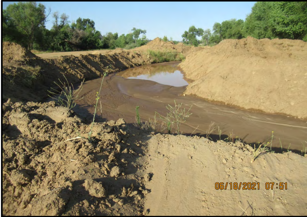
Constructed wash-water ditch in the east part of the site, looking southwest; 06/18/21. This ditch carries wash water from the mine in to the quarry pond.
