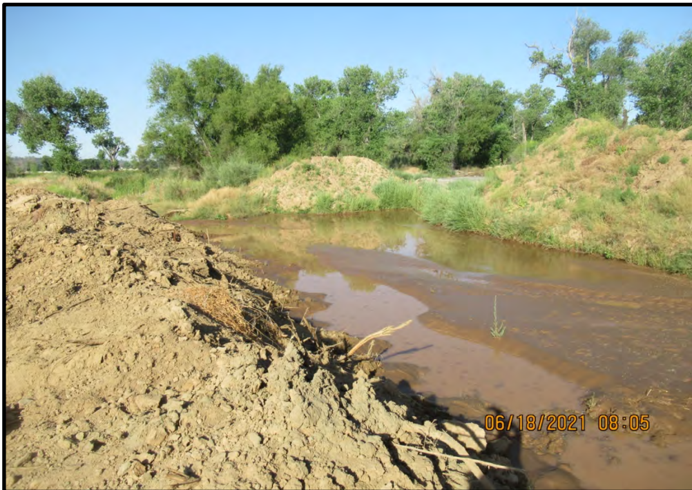
Constructed ditch just downstream of the previous picture, looking southwest from the east part of the site; 06/18/21. This ditch was constructed in uplands for mining operations.
